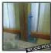
REPAIR ROTTEN POSTS
